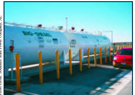
Photo credit: Southern States Power Company, AZ
