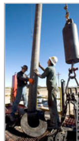
Workers install a pipe in a geothermal water well at Raser Technologies' Thermo
