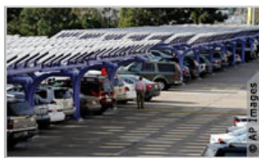
Growing demand for solar systems, such as this one at the Department of Water and Power in Los Angeles, will require more installers.
